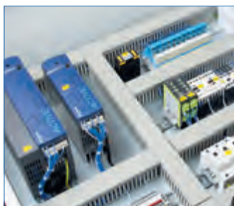
Frequency converter-control system
